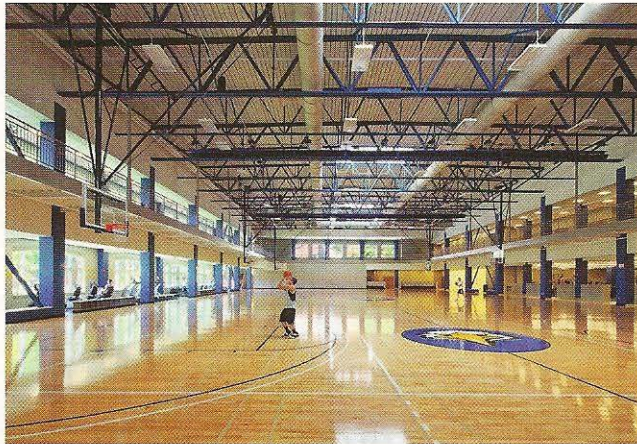
Lighting controls take cues from the daylight to determine how much power should be used.
